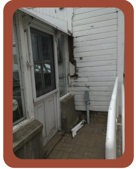
Wood rotting on the Interpretive Center prior to the Lifecycle Renewal
